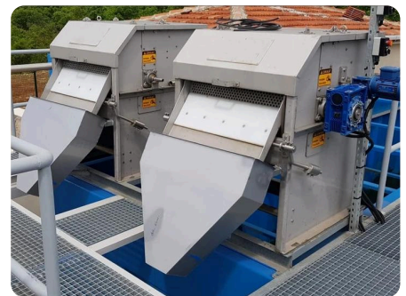
Water treatment equipment
