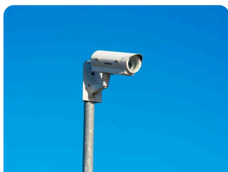
Security and fire detection
