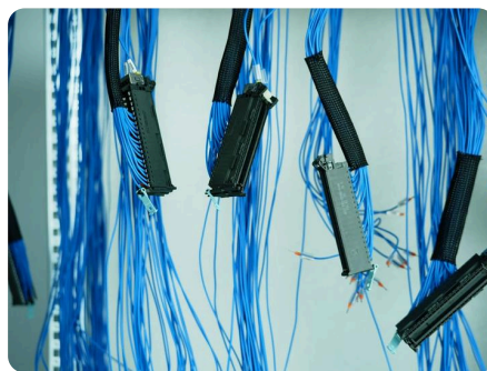
Signal and control cable
