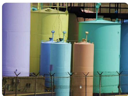
Polyethylene water tank
